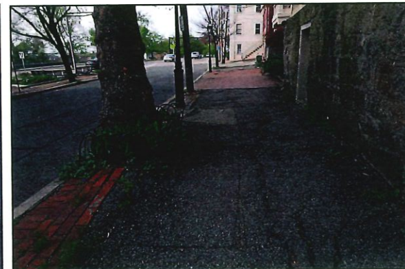
Poor Surface: Buckled and broken paving.
