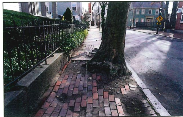
Impassable: Inadequate clearance and dislodged paving.
