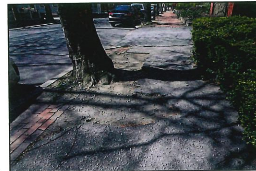
Very Poor Surface: Broken and missing paving.
