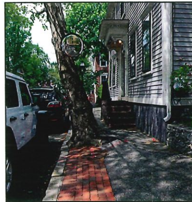
Impassable: Inadequate clearance and buckled paving.
