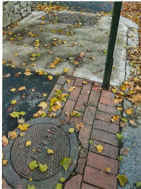
Brick border unnecessarily replaced by concrete
