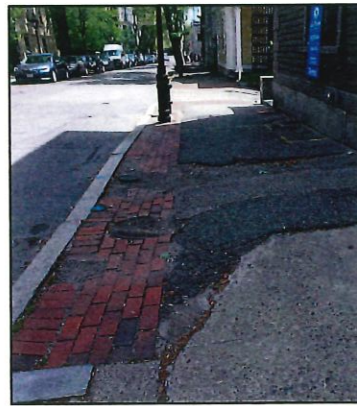
Poor Surface: Broken and missing paving.
