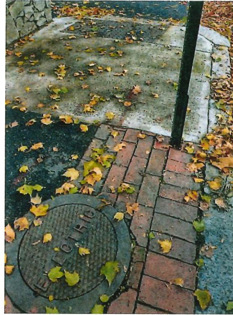
Brick border unnecessarily replaced by concrete
