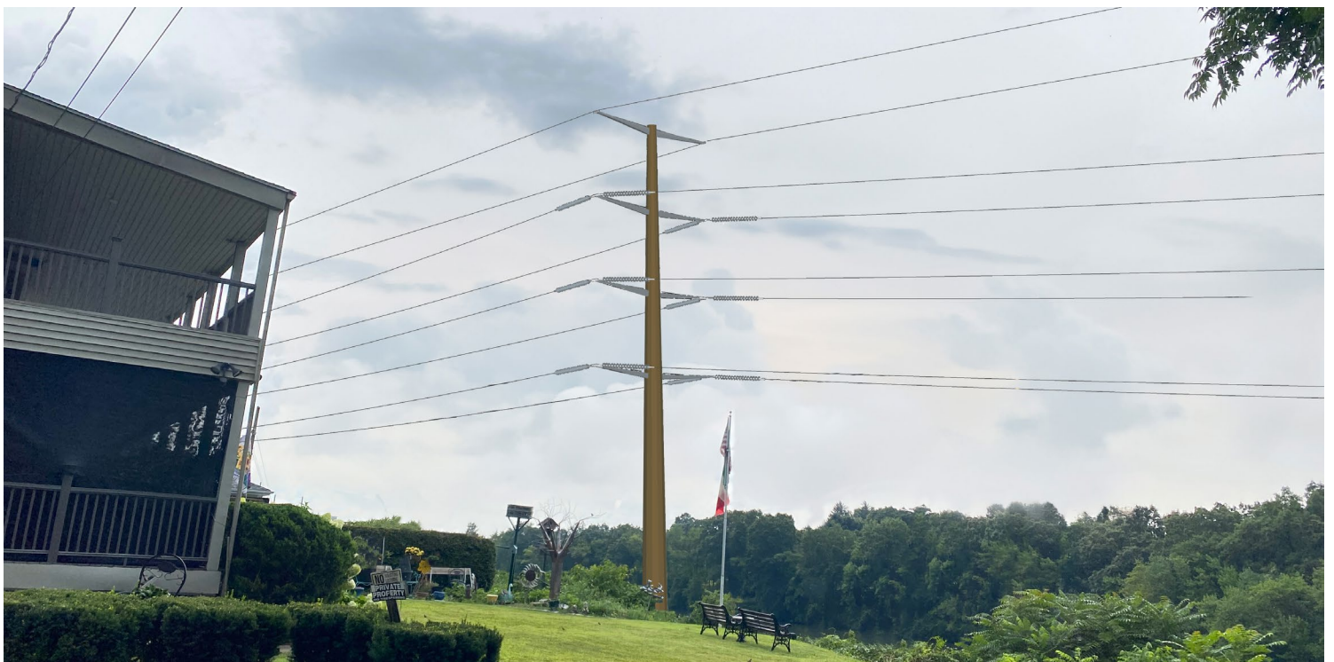
Photo #2a: Visual sim of the proposed line 'Q143S/ R144'. Here is showing Q143S, Structure 132 with weathered steel.
