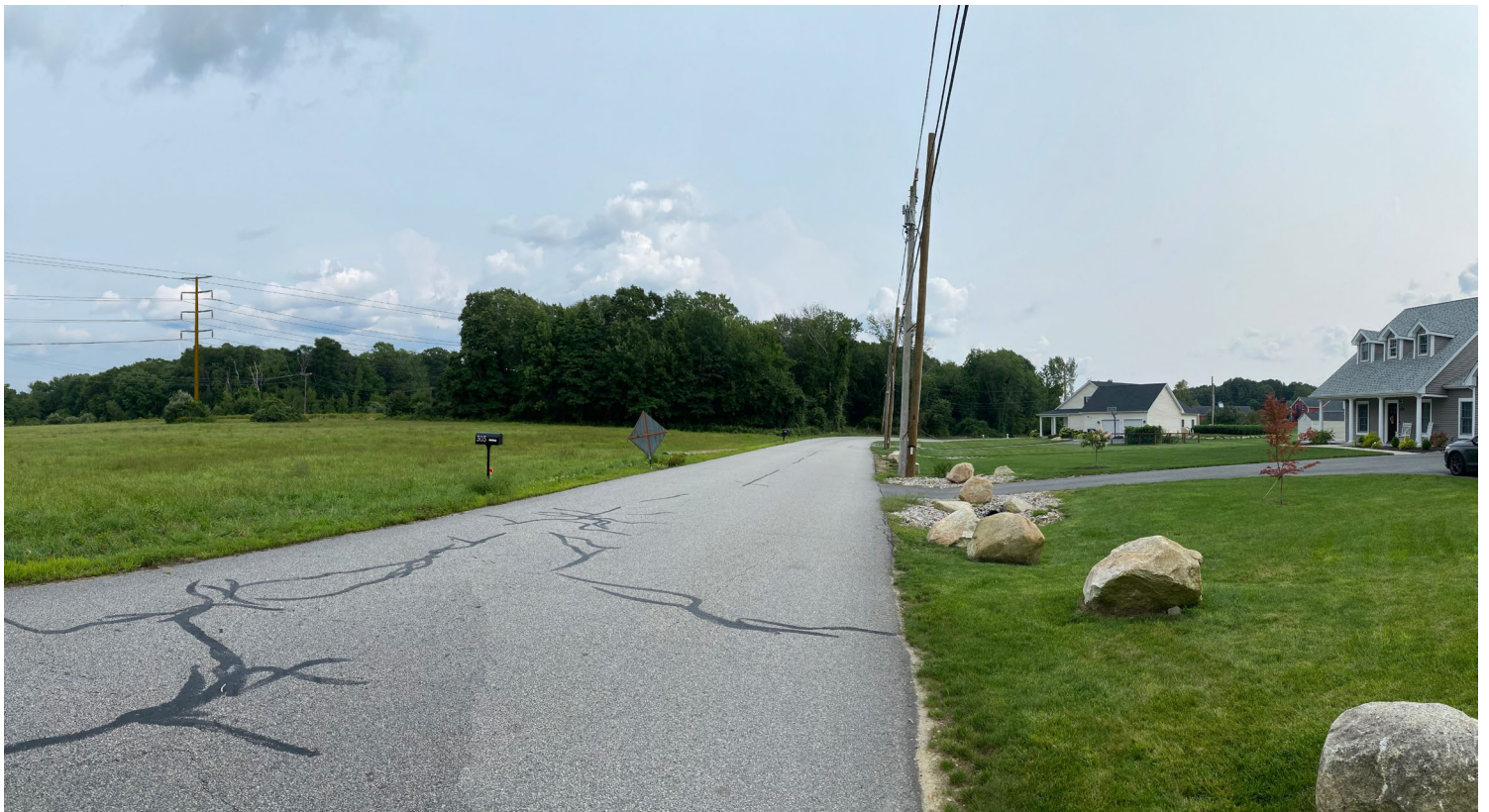
Photo #1a: Visual sim of the proposed line 'Q143S/ R144'. Here is showing Q143S, Structure 28 with weathered steel.
